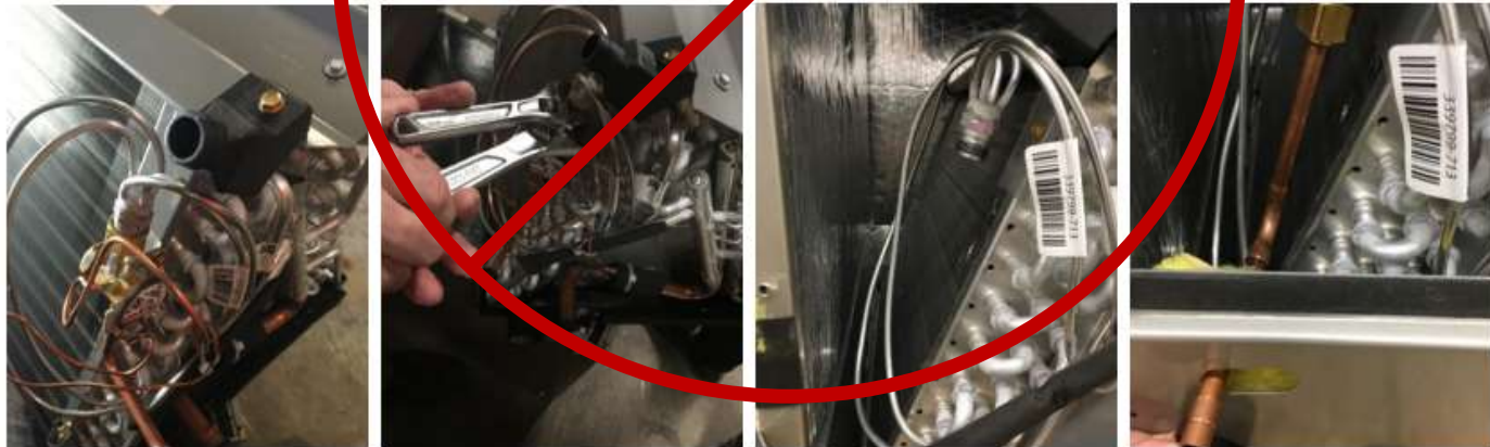
Fig. 14 — Piping Adapter Replacement
