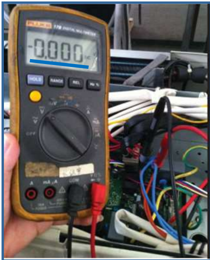
Cooling Mode De-energized
