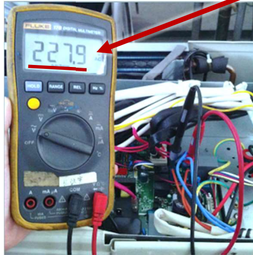
Heating Mode Energized
