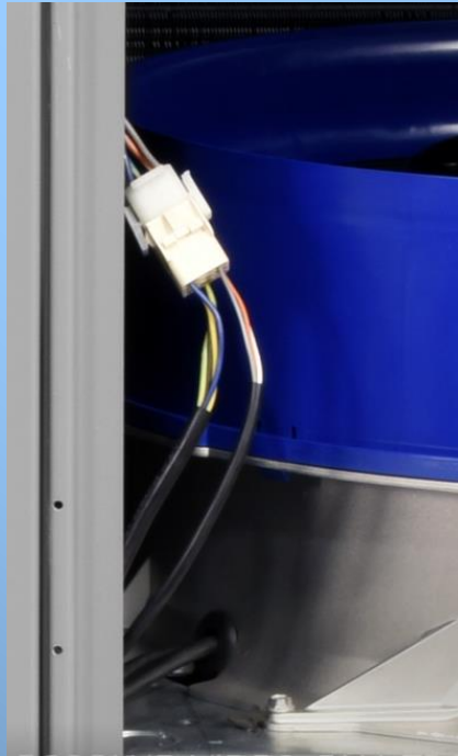
Plug location in the blower section
