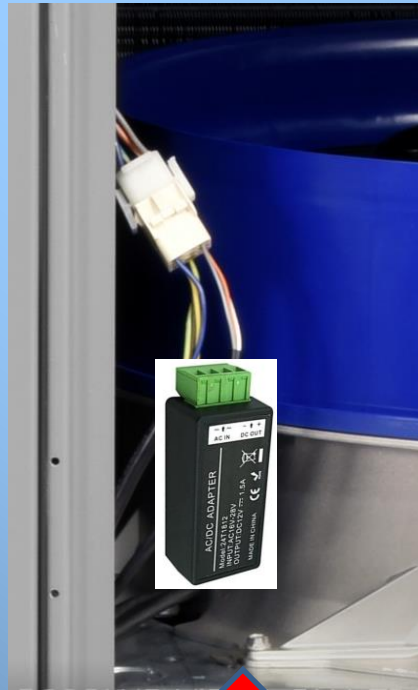
Plug location in the blower section
